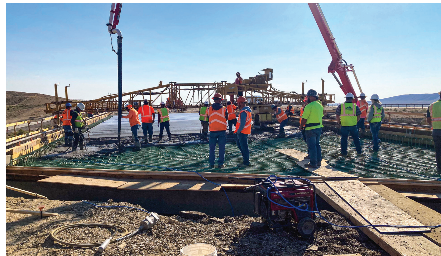
A crew with IHC Scott work on pouring concrete for a bridge deck at the Baxter Interchange on I-80 east of Rock Springs. The contractor and WYDOT were awarded an Excellence in Concrete Paving award this year by the Colorado/Wyoming chapter of the American Concrete Paving Association.
