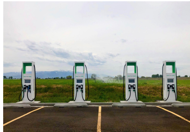
Figure 7: Electrify America EV charging stations along I-84 outside Heyburn, Idaho.
