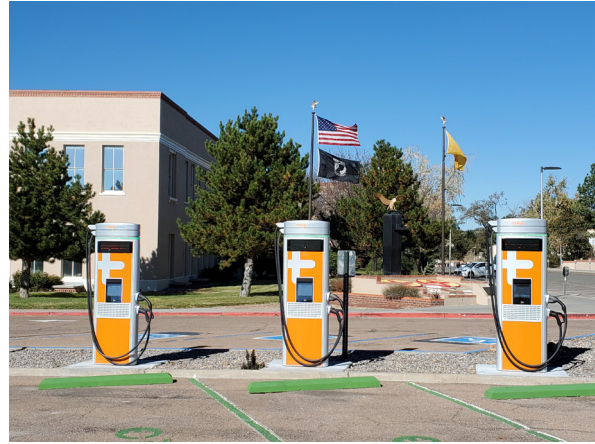
Figure 9: EV charger stations located at the New Mexico State Capitol in Santa Fe, New Mexico.
