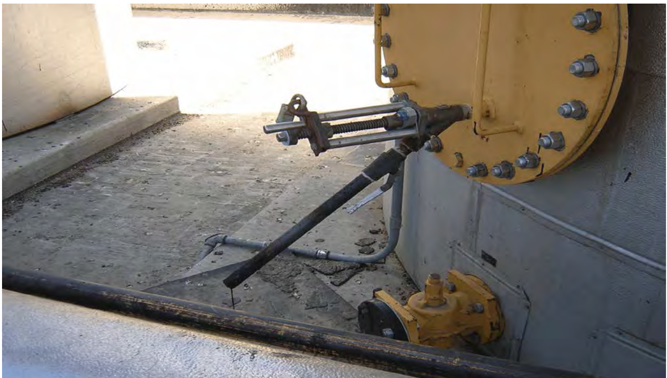
Figure 2 - Typical Sampling Valve for Storage Tank
