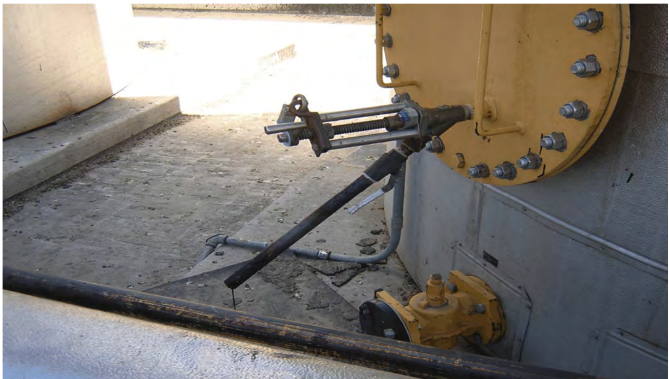
Figure 2 - Typical Sampling Valve for Storage Tank
