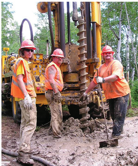
Using the three WYDOT drill rigs and backhoe, Geology completed 484 test holes and 8,362 feet of drilling and digging for subsurface investigations.
