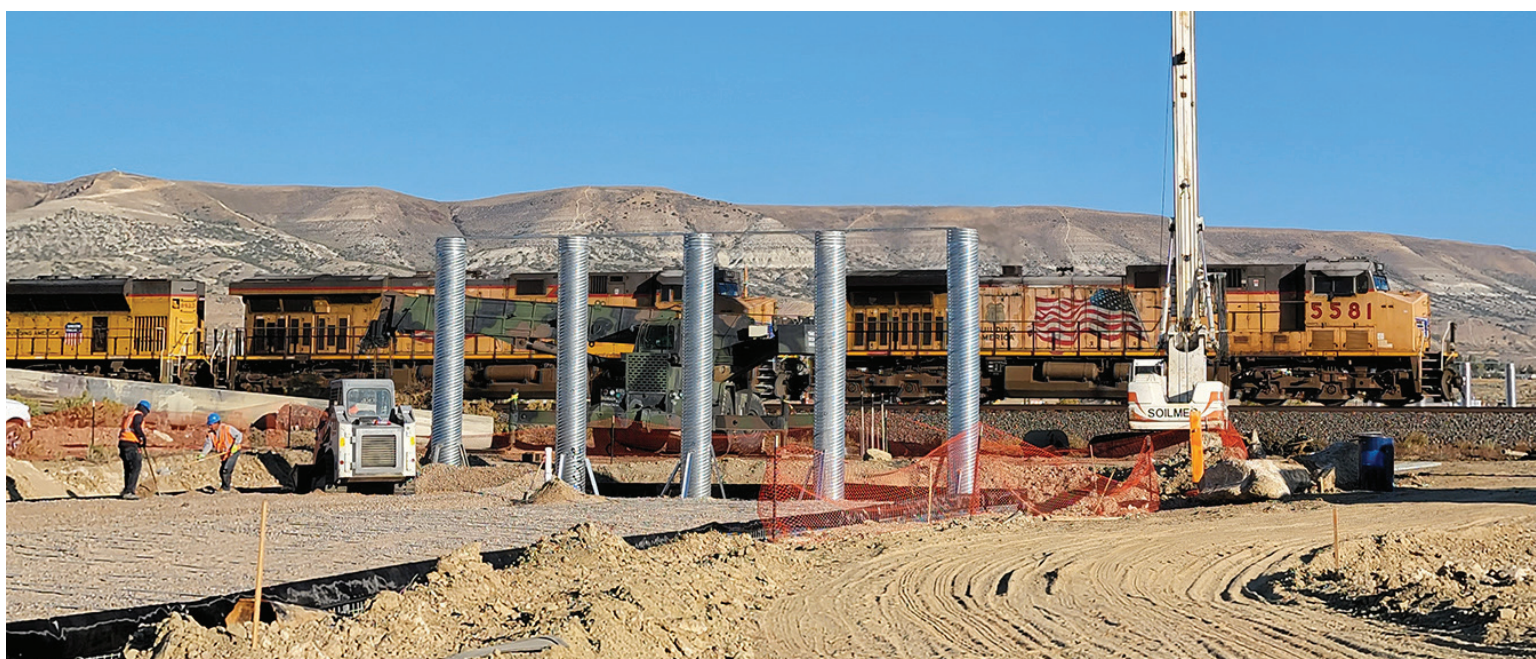
D3 partnered with city and county agencies on Interchange Road, and the project is slated for 2023 completion.
