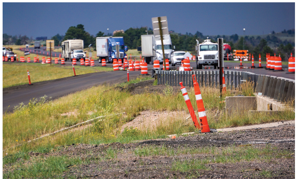
Road construction zones lined with traffic control on I-80 during a paving operation.
