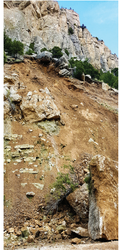
A rock slide in Wind River Canyon was cause for repair on WYO 789/US 20.
