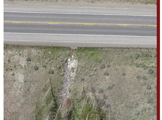
SURVEYS and district staff used an unmanned aerial vehicle to collect nearly 750 photographs of the Red Roof Slide along US 280.
