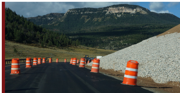
For the Chief Joseph Scenic Highway landslide remediation, GEOLOGY and the contractor approved a value engineering proposal involving changes to the ground improvement design and saving about $133,000.
