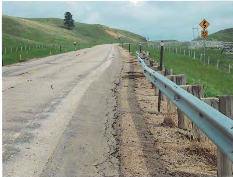
Figure 2: West lateral margin showing offset of road due to movement of the Rupe Hill Landslide.
