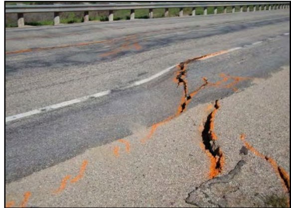
Figure 1-3. Rupe Hill landslide along US 14 at milepost 197.4 May 2011
